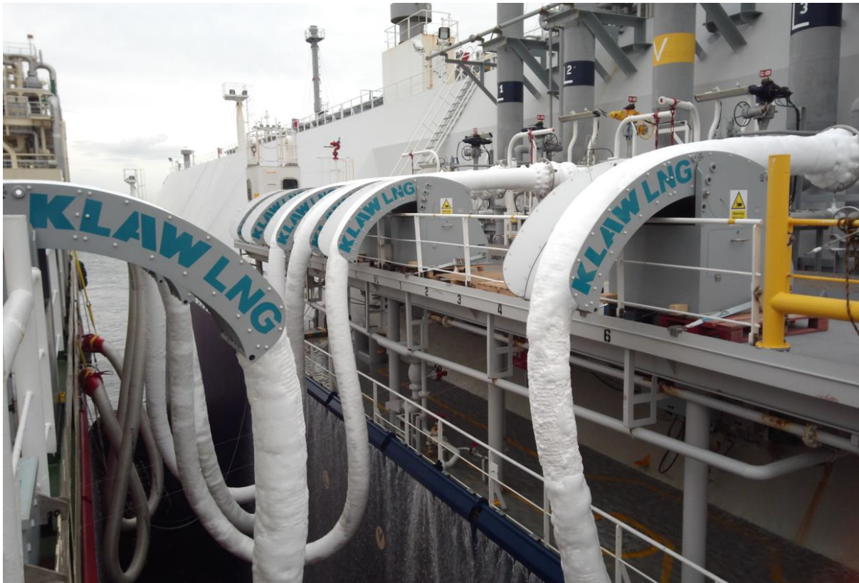
Figure 10 Flexible Hoses during Cargo Operation
