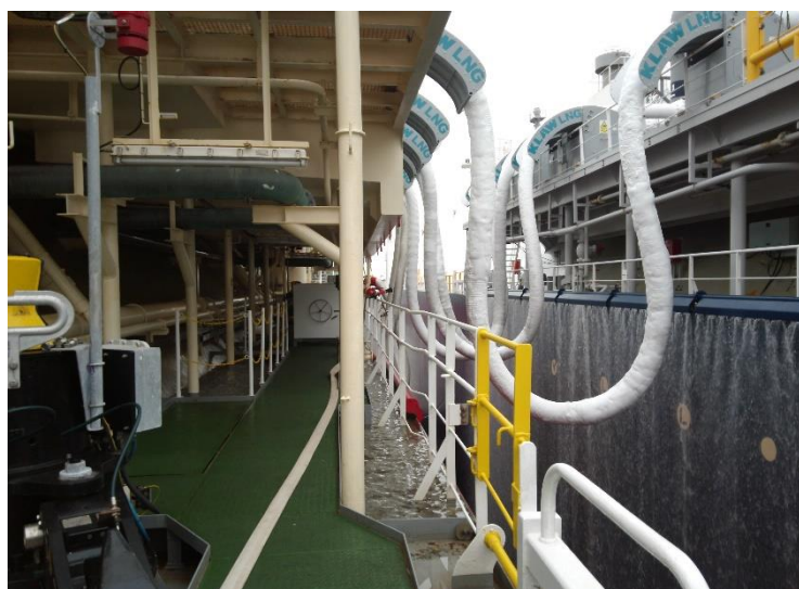
Figure 34 Water Curtain / Deluge
