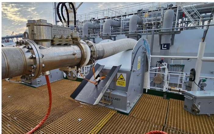
Figure 17 Fall Arrest system on the FSRU
