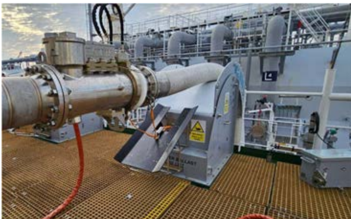
Figure 15 Fall Arrest system on the FSRU
