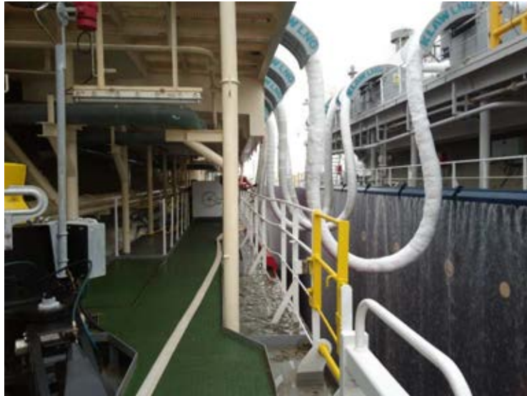
Figure 32 Water Curtain / Deluge
